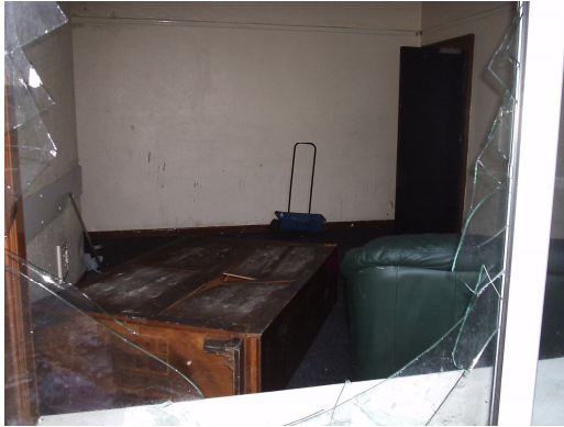
Picture 1 showing a Broken Window.
